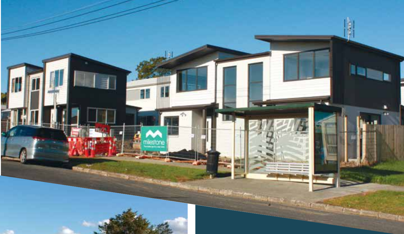
These 11 new homes on Fenchurch Street for HNZN will be ready for tenants by early July
