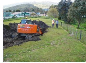
Breaking new ground for Abbeyfield's new development in Greymouth. Read the full media release above.
